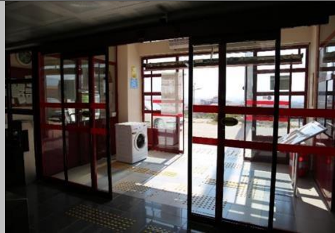
Automatic Opening Doors
