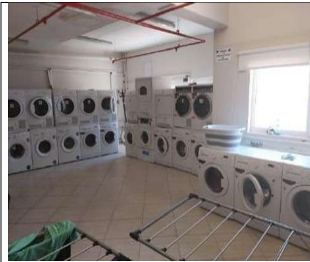
Washing machines and tumble dryers (Kütahya Dumlupınar University, Turkey)
