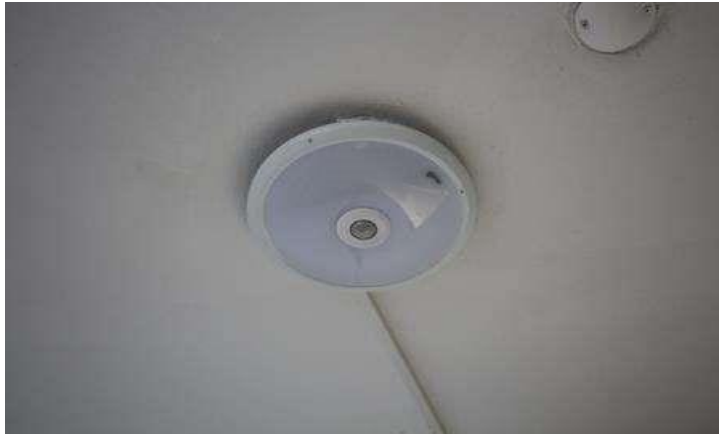
Sensors (auto lighting control) (Kütahya Dumlupınar University, Turkey)
