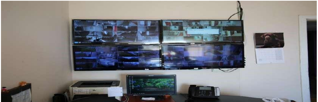
Security Video Monitoring System (Kütahya Dumlupınar University, Turkey)
