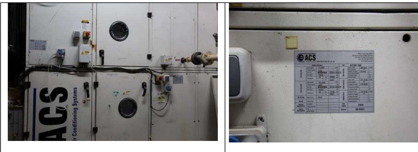
Air Quality (Fans) (Kütahya Dumlupınar University, Turkey)
