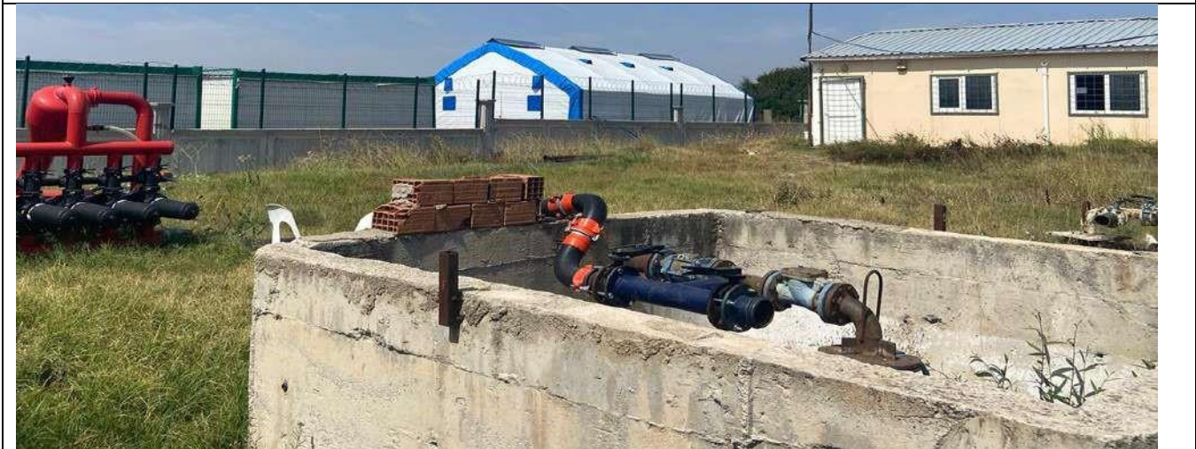
Rainwater Collection Tank (Kütahya Dumlupınar University, Turkey)
