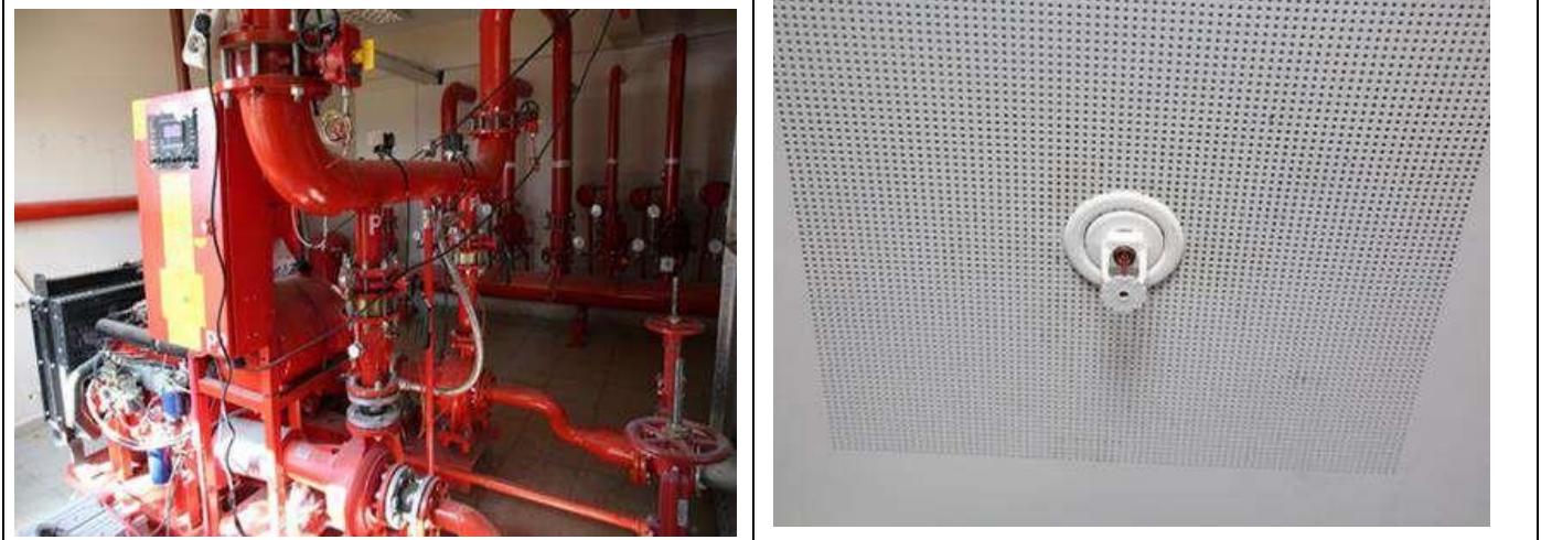
5.Fire Extinguishing System (Kütahya Dumlupınar University, Turkey)
