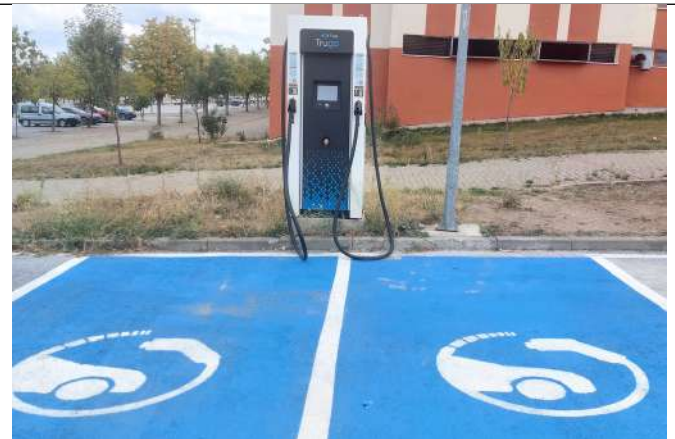
Electric Vehicle Charging Station (Kütahya Dumlupınar University, TURKEY)
