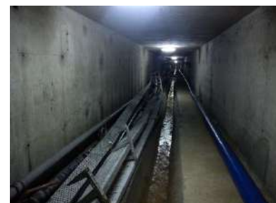
Underground transmission lines (rainwater outfall, center)
