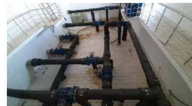
Storage main valve lines
