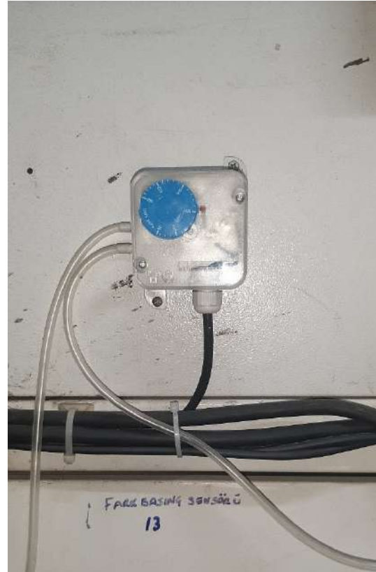
Air Handling Unit Sensor Example
