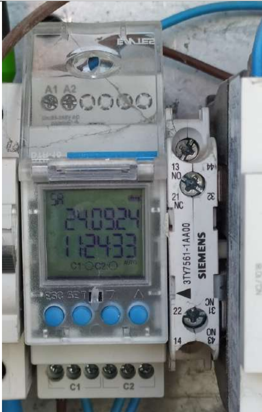
Smart Lighting Control
