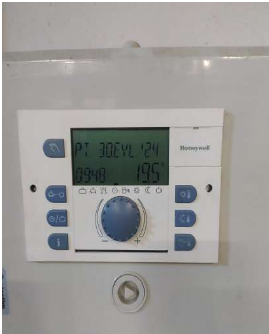
Heating Installation Automation
