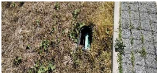
Typical High Water Efficiency Timer And Drip Irrigation System Used Throughout The Campus
