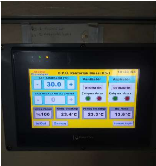
Air Handling Unit Control Panel Example
