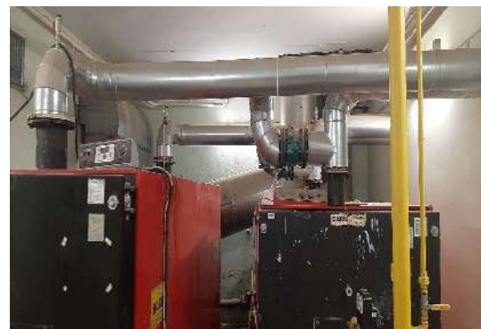
High Efficiency Heating System Equipment
