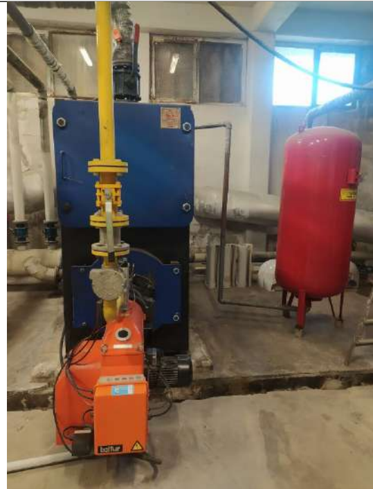
High Efficiency Heating System Equipment
