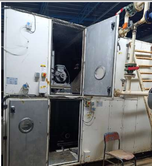
Whole System Air Handling Unit Examples
