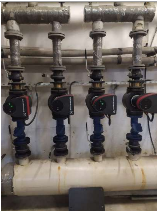
High Efficiency Heating System Equipment
