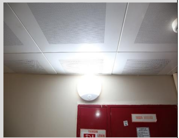
Led lights (high efficiency)
