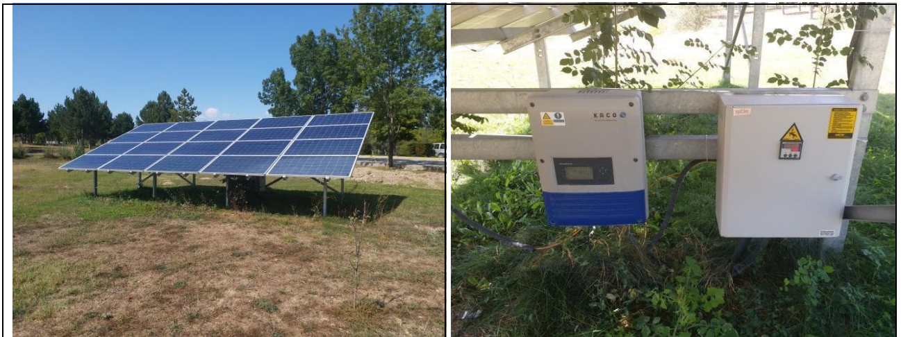
5Kwh Solar PV energy system connected to campus electrical grid.
