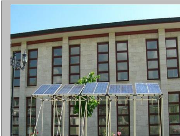
Solar panels (Dumlupınar University, Turkey)
