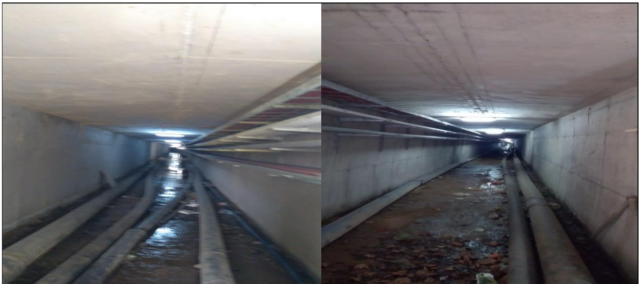
Hot water channels leading to Physiotherapy -Rehabilitation Hospital and Olympic Swimming Pool (Kütahya Dumlupınar University, Turkey)
